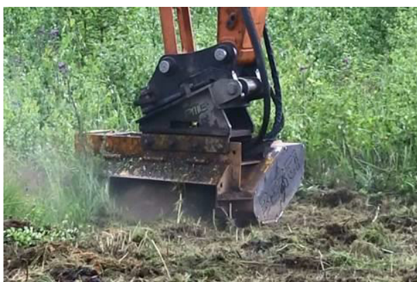
Figure 6. Milling the topsoil (stumps, roots, small sticks, grass etc.) for working platform.
