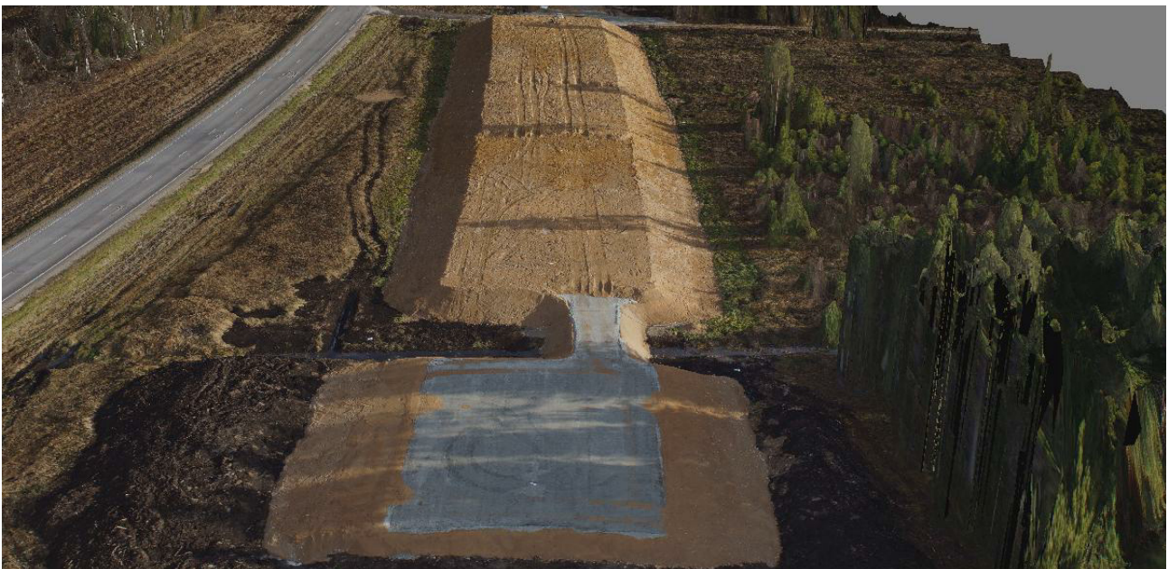
Figure 13. 3D surface model created from the RPAS photos combined with aerial photos (Julge 2015). Surface after construction of surcharge loading 5.11.2015 (RPAS=Remotely Piloted Aircraft System).
