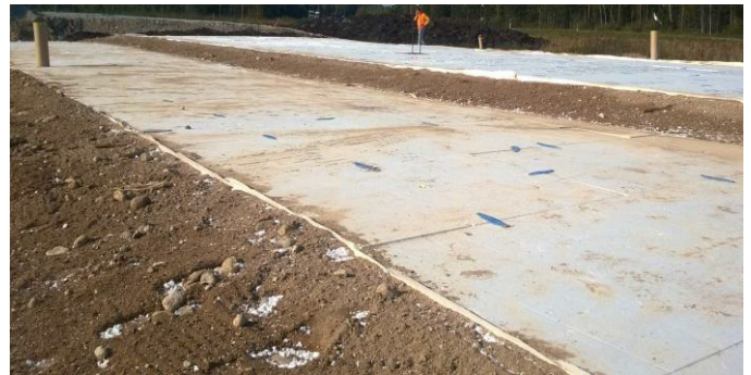
j) Surface of the EPS-layer at sec. 5. Plastic connectors on between EPS-blocks (24.9.2015)
