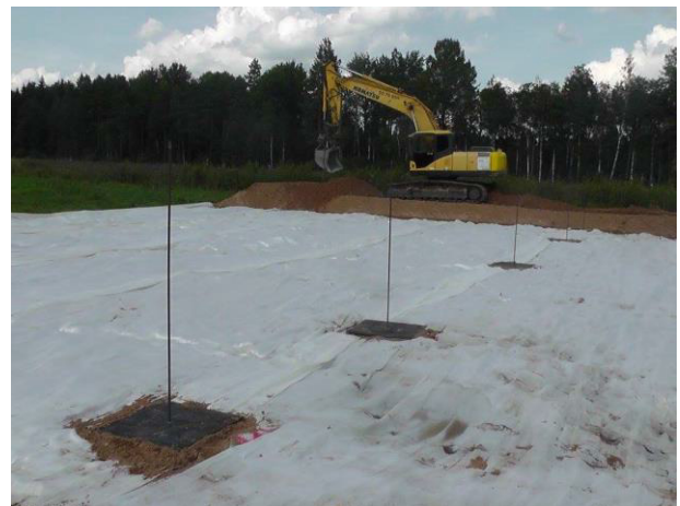
Figure 15. Peat roads placed in pre-designed locations on top of the geotextile-covered peat layer. (Ellmann 2015)
