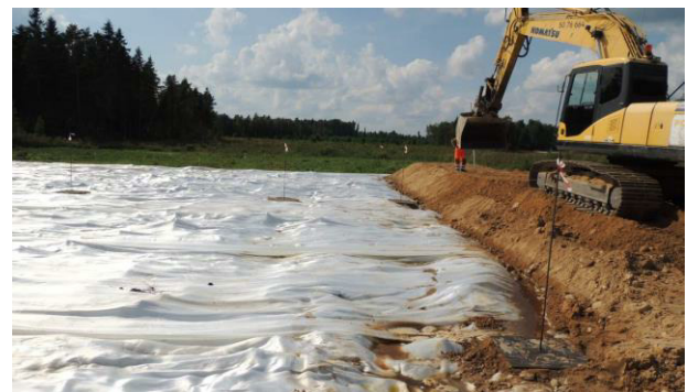
f) Construction of edge barrier at sec. 4. Peat rod in bottom right corner. (12.8.2015)
